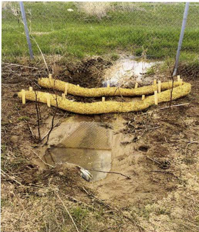
Photo submitted by applicant on May 3, 2019 of installed BMPs at outlet to the Right-of-Way
